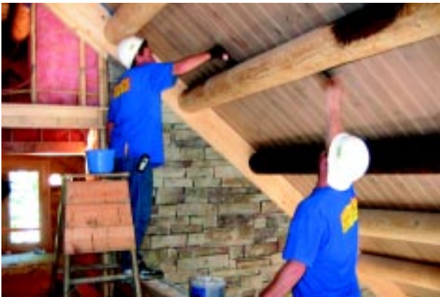
Application of Lifeline™ interior stains on ceilings, log beams and interior log walls
