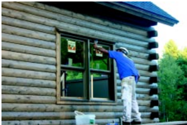
Volunteers applying Lifeline Ultra-2™ stain to the exterior walls of the Goodale log home
